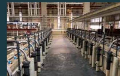
KTL & pretreatment 12 immersion processes for chemical cleaning and subsequent KTL coating
